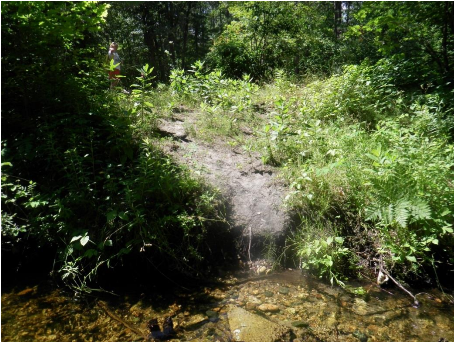
Figure 24: Erosion on Elliot Creek (DGB 03)
