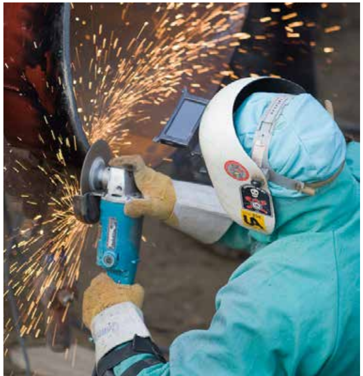
Welder is conducting pipeline repair as part of Enbridge’s Integrity Management Program.
