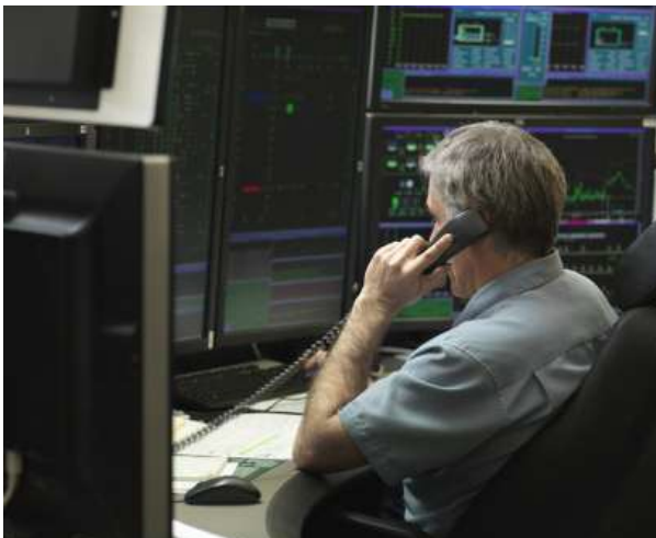
Pipelines, including Line 5, are monitored around the clock by operators in our state-of-the-art control center
